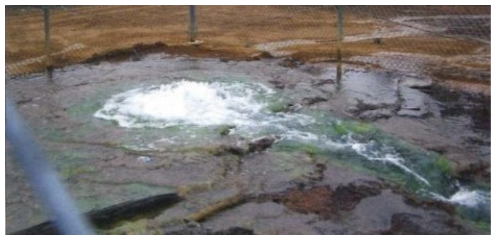
Hughes Borehole impacting the Little Conemaugh River.
