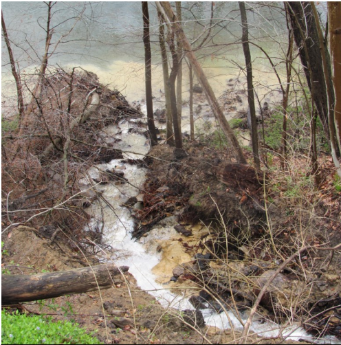
The outflow of sediment-laden water along a hillside overlooking the Stonycreek River at Hollsopple.
